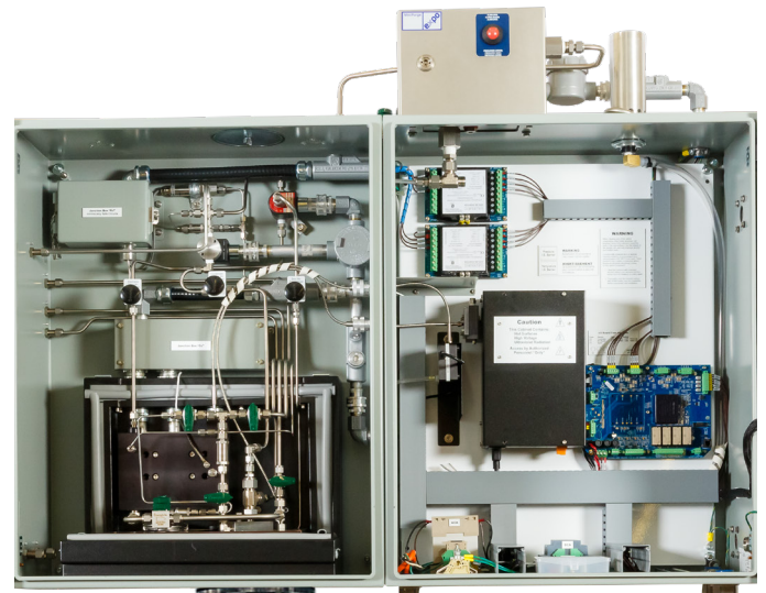
Note: Photo With Cabinet Doors Open
