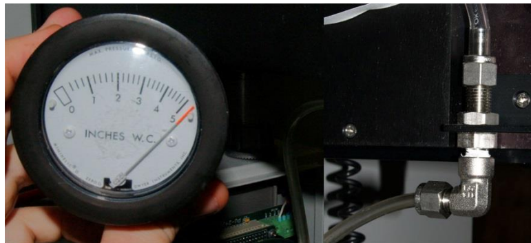
Figure 3-24: Minihelic Indicating a Good Seal (L); Connected to Vent Elbow (R)
