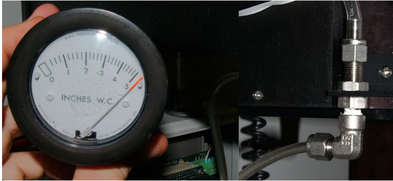
Figure 3-21: Minihelic Indicating a Good Seal (L); Connected to Vent Elbow (R)
