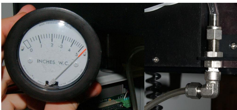
Figure 3-23: Minihelic Indicating a Good Seal (L); Connected to Vent Elbow (R)
